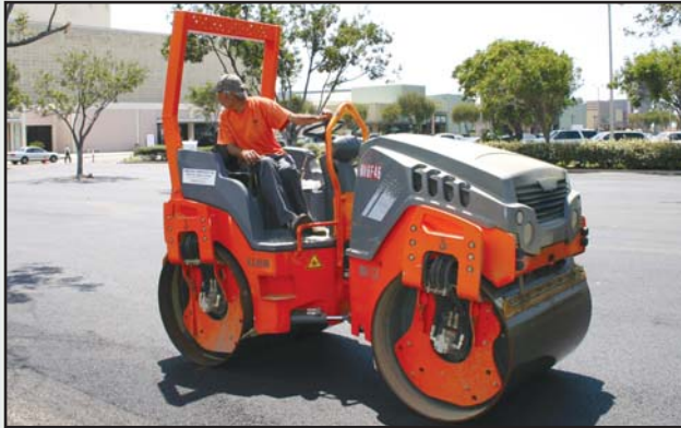
Century Paving, Inc.'s new Hamm HD 13 compacting a parking lot at the Chula Vista Center Mall.
